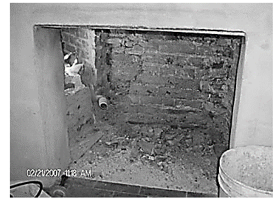
Badly Deteriorated Firebox
