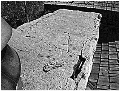
Damaged Chimney Cap
