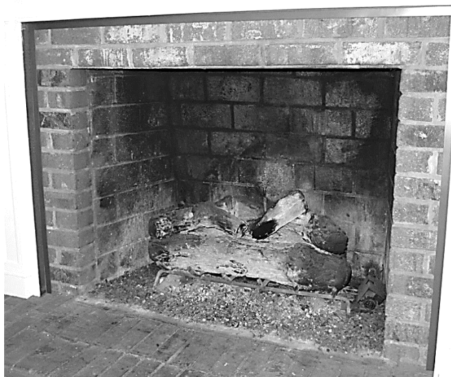
Masonry Woodburning Fireplace
